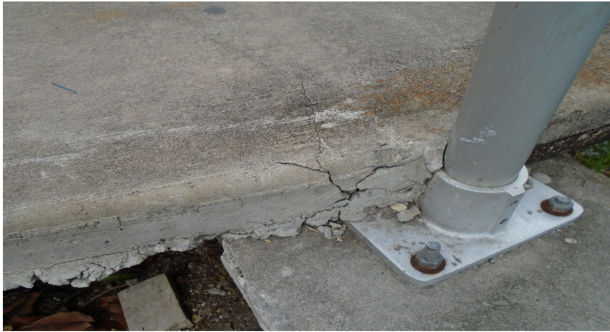
Significant cracks present in concrete slab
