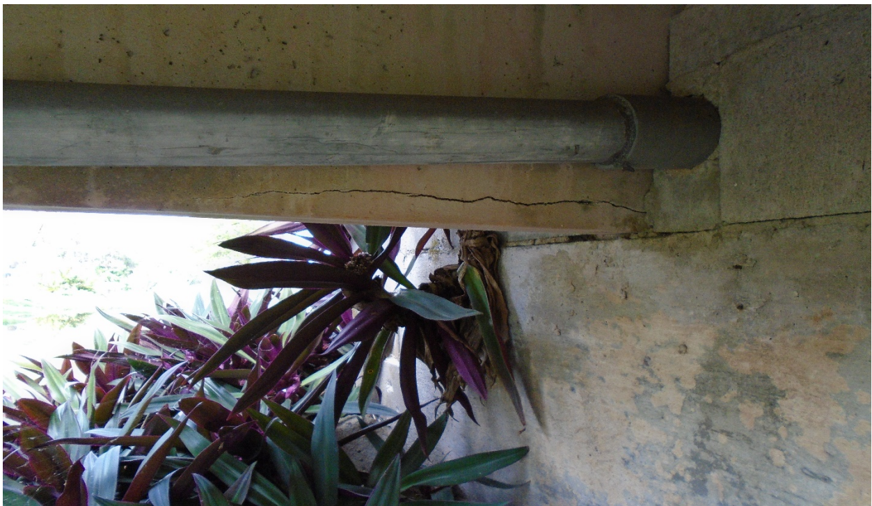
Significant cracks is concrete supporting beam
