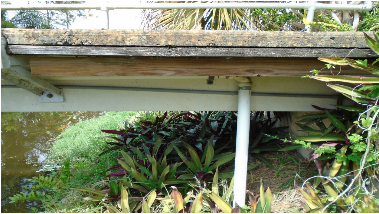
Photo depicting attempted repairs for support of bridge
